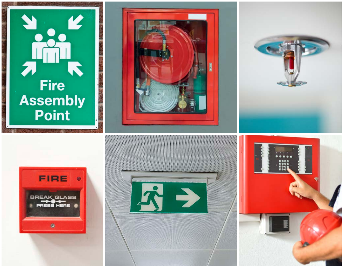
Figure 3.1. Examples of Fire and Life Safety Equipment and Signage (clockwise from top left): Assembly Point Sign, Fire Extinguisher inside Hose Reel Cabinet, Automatic Fire Sprinkler, Fire Alarm Control Panel, Exit Sign, Fire Alarm Call Point
